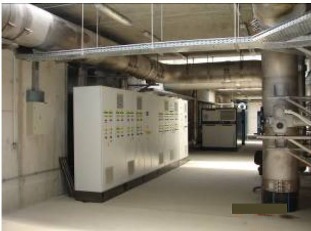
Control unit of blowers and other motor drives
